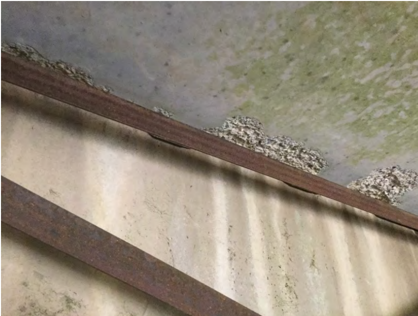
Damage noted to underside of panel 1 at left bank
