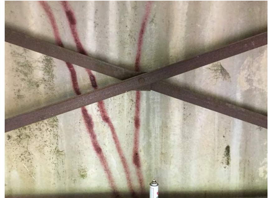
Hairline cracks noted on left bank ballast wall
